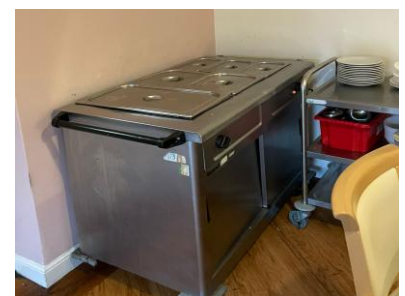
Hazard: Bain Marie with no hazard notice
